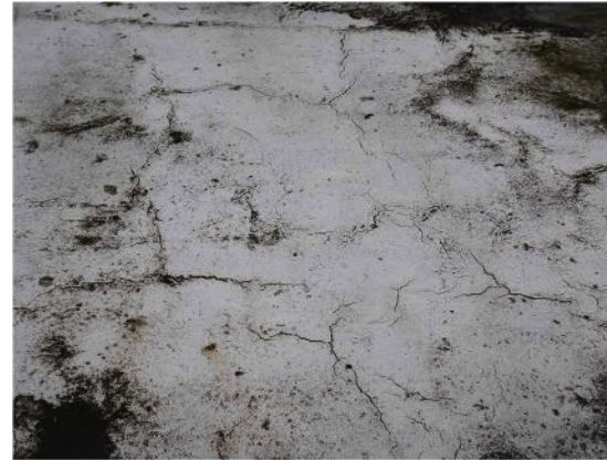
A close-up of the asphalt roof, showing cracks
