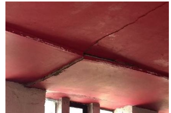
Damage to ceiling in church due to water leak
